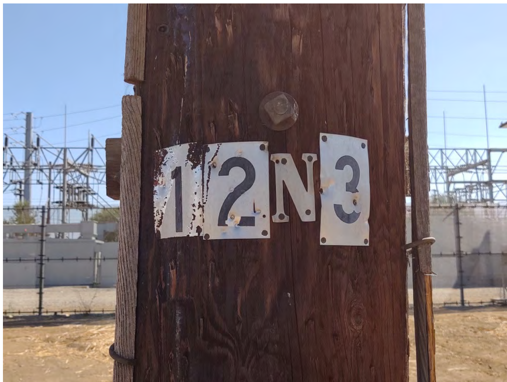
Power Pole 12N3. View to east
