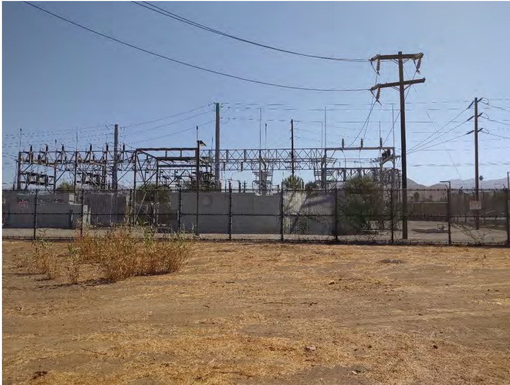
Eastern Parcel and Hunter Substation. View to east
