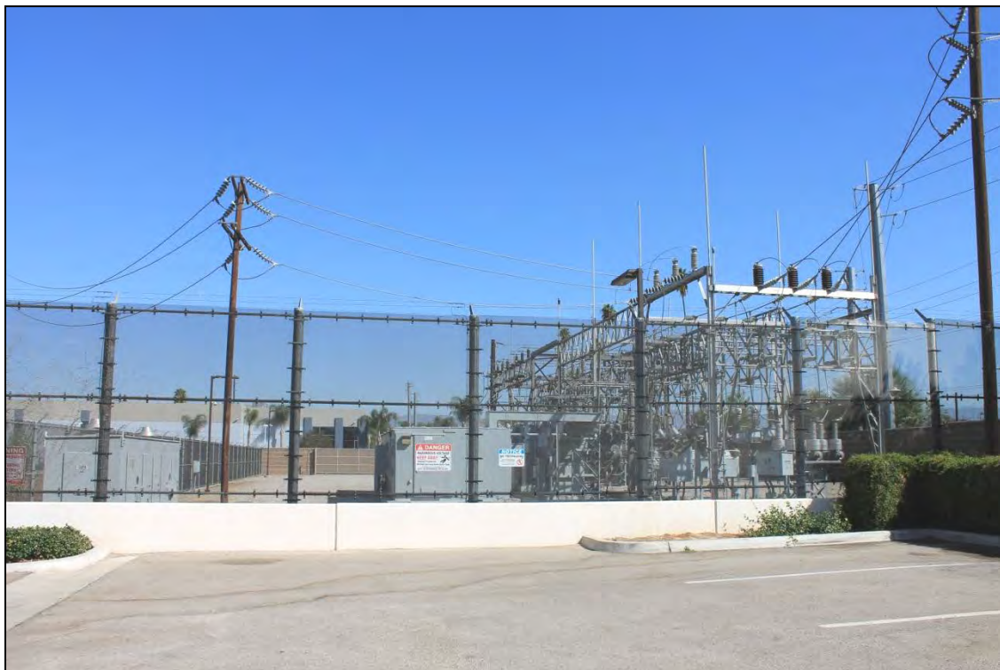
Figure 4: Hunter Substation. View looking north.
