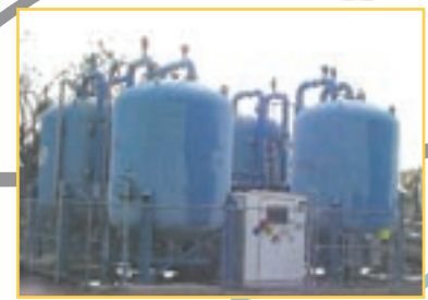
TCE Treatment Plant
