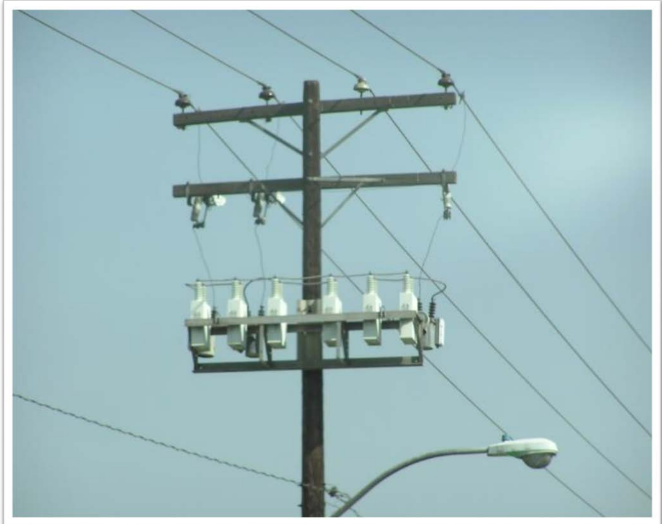
Capacitor Bank & Streetlight
